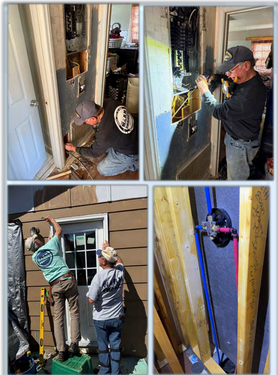
Members of Post 193 utilized some of the funds donated by Chapin's Post 193 American Legion Riders to install water and electric lines for a washer & dryer, rewire the service panel, repair a dishwasher, and install a exterior door for a single mother's home that was severely damaged during Hurricane Helena. (25 March 2025, Swannanoa, NC)
